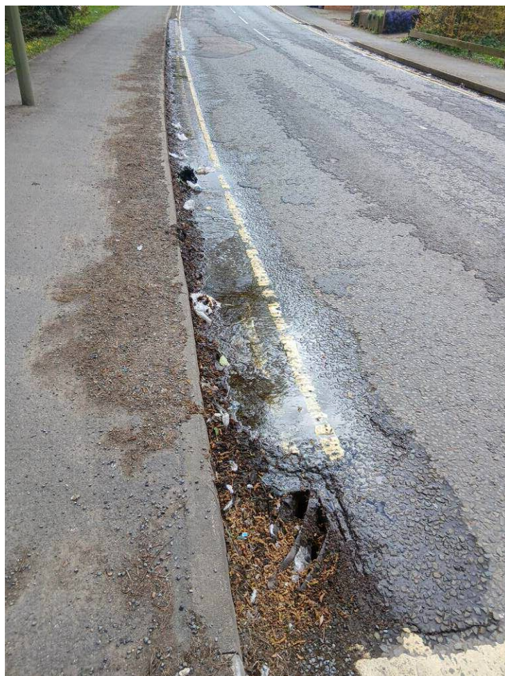
Flooded Drains – Hightown Road
